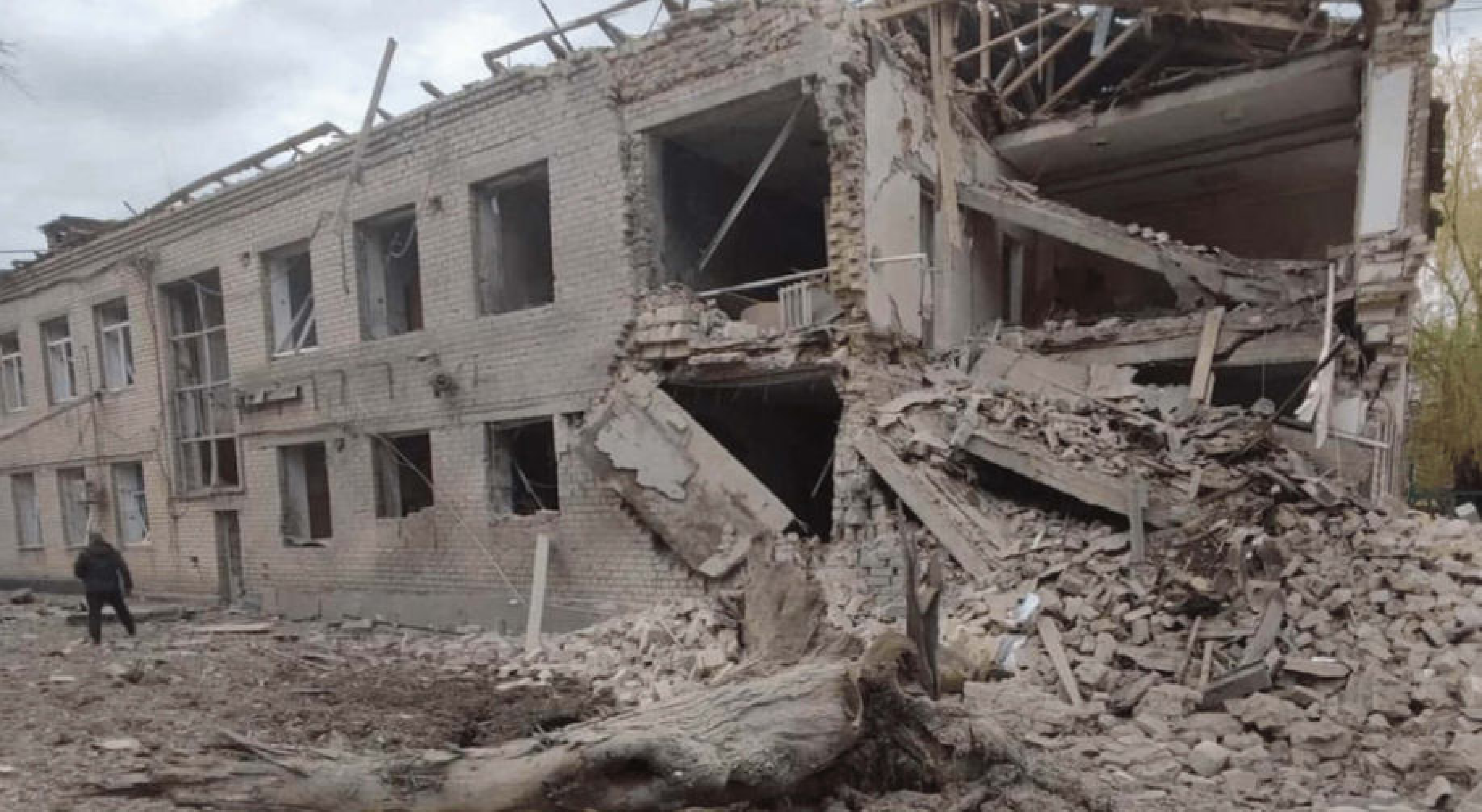
The aftermath of an artillery strike on the hospital in Bashtanka (Mykolaiv region), photo: Hanna Zamazieieva, 04/19/22
